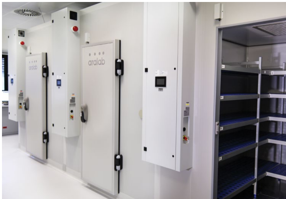
STABILITY ROOMS TURNKEY PROJECT BY ARALAB
