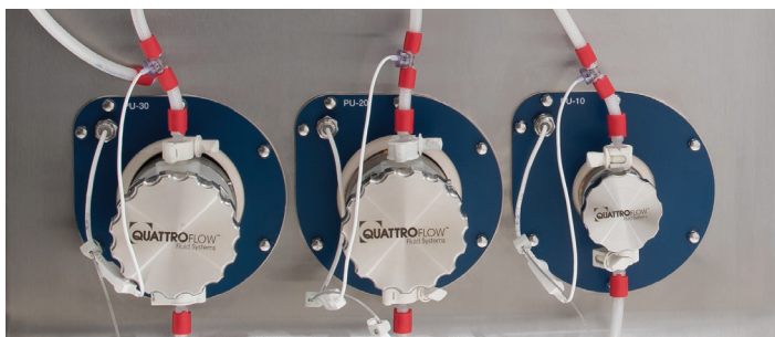
Figure 5. Three positive displacement pumps.
