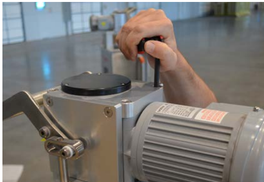
Figure 3.16. Removing one of the four bolts from the top of the motor assembly.
