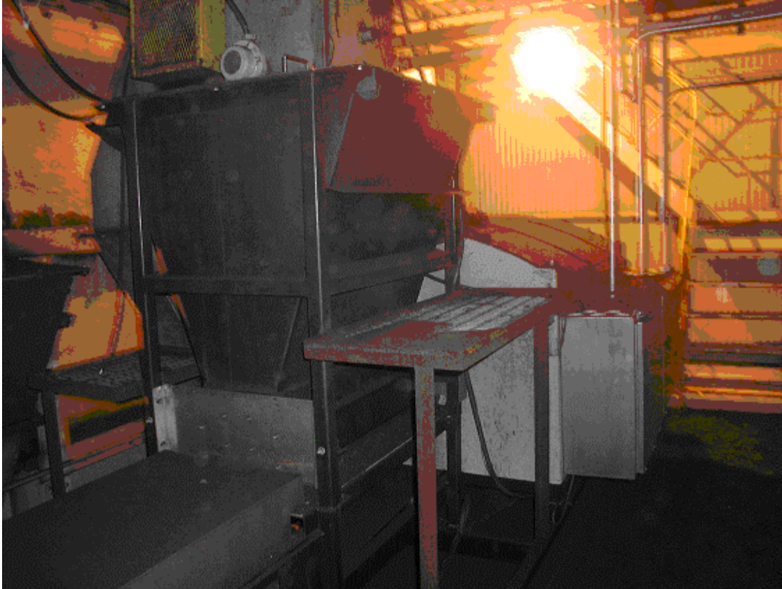
Figure 4. Gamma-Metrics CQM Coal Analyzer in Loadout Tower
