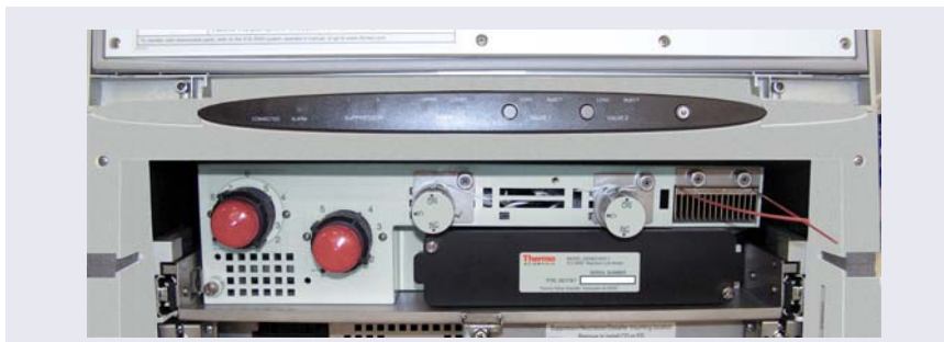
Figure B-26. DC with AM Installed
