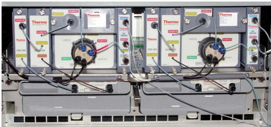
Figure 4-19. Completed IC Cube Plumbing for a Dual Conductivity Detection System
