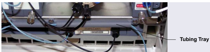
Figure 4-18. IC Cube Tubing Trays (System #2 of Dual System Shown)
