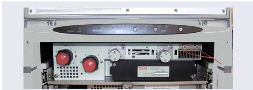
Figure B-28. DC with AM Installed
