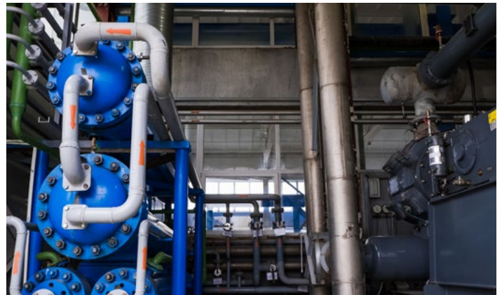
Thermo Scientific Systems Water-to-Water Heat Exchanger
