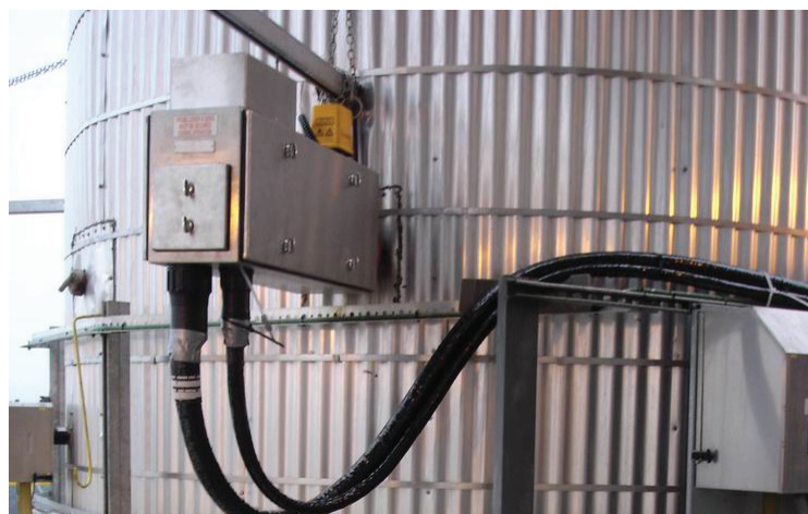
Figure 1 View of the Model 83i Probe at southeastern cement kiln.
